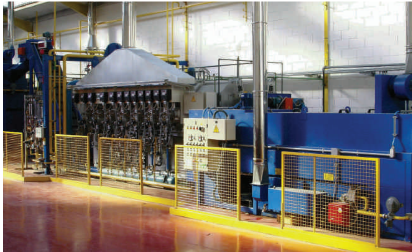
▲ Sib Societa' Industriale Bagnolo manufactures heat treatment systems
