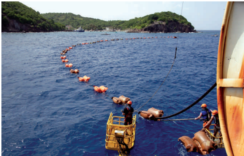
▲ Nexans will provide the subsea power link to connect Hainan Island to the Chinese mainland
