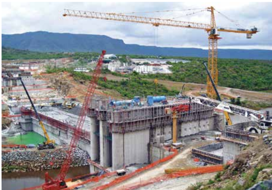
Potain tower cranes have moved material on many important civil engineering projects in South Africa.
