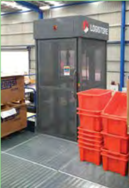
Logistore Goods Hoist upper level entrance
