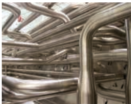
Sanitary piping is stainless steel high purity tubing for biopharmaceutical, food and beverage facilities. Whilst the focus had always been structural integrity, the issue of hygienic joints introduced new fabrication challenges to allow the systems to be cleanable and eliminate bacterial entrapment areas.
