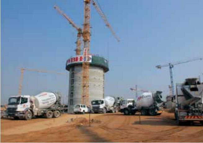
As the concrete supplier to this complex project, AfriSam designed 19 project-specific and special application mixes.
