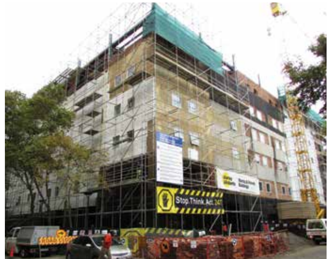
ABOVE: The project site is bordered on three sides by public roads.
