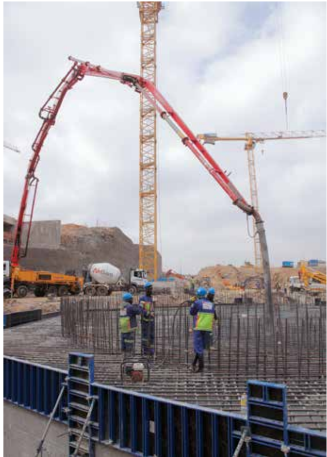
Concrete is poured continuously within shutters and the system is lifted incrementally as concrete is poured, creating a structure without joints.
