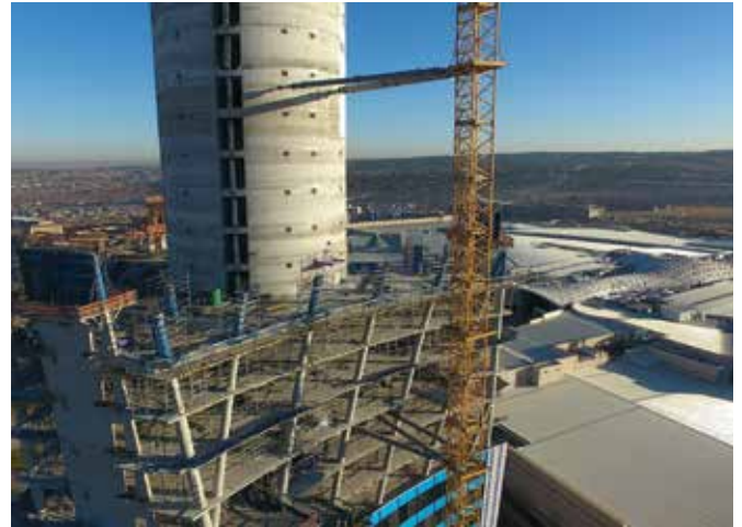
The core wall, at a height of 118 metres and thickness of 450 mm, was constructed using an interesting method of construction – slip forming.
