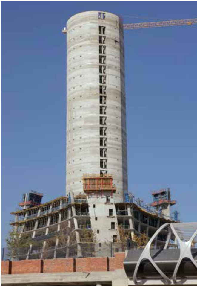
Visible from a 30 km radius, the R1,5-billion PwC Tower will comprise 45 000 m 2 of office space and house 3 500 employees.
