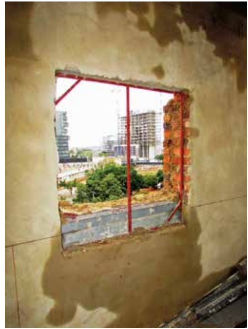
Sub-frames are being used for all of the openings in the external walls to ensure they are consistent to the mm.
