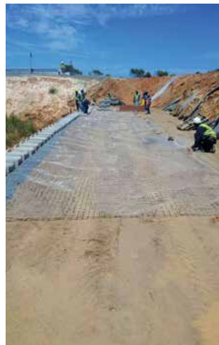
The substation, which consists of a 400/132 kV high voltage yard gave the Eskom Engineers some initial challenges, including a large cut to fill operation necessary to create a level platform for the new transformers. This necessitated the erection of a large peripheral precast segmental block retaining wall system.
