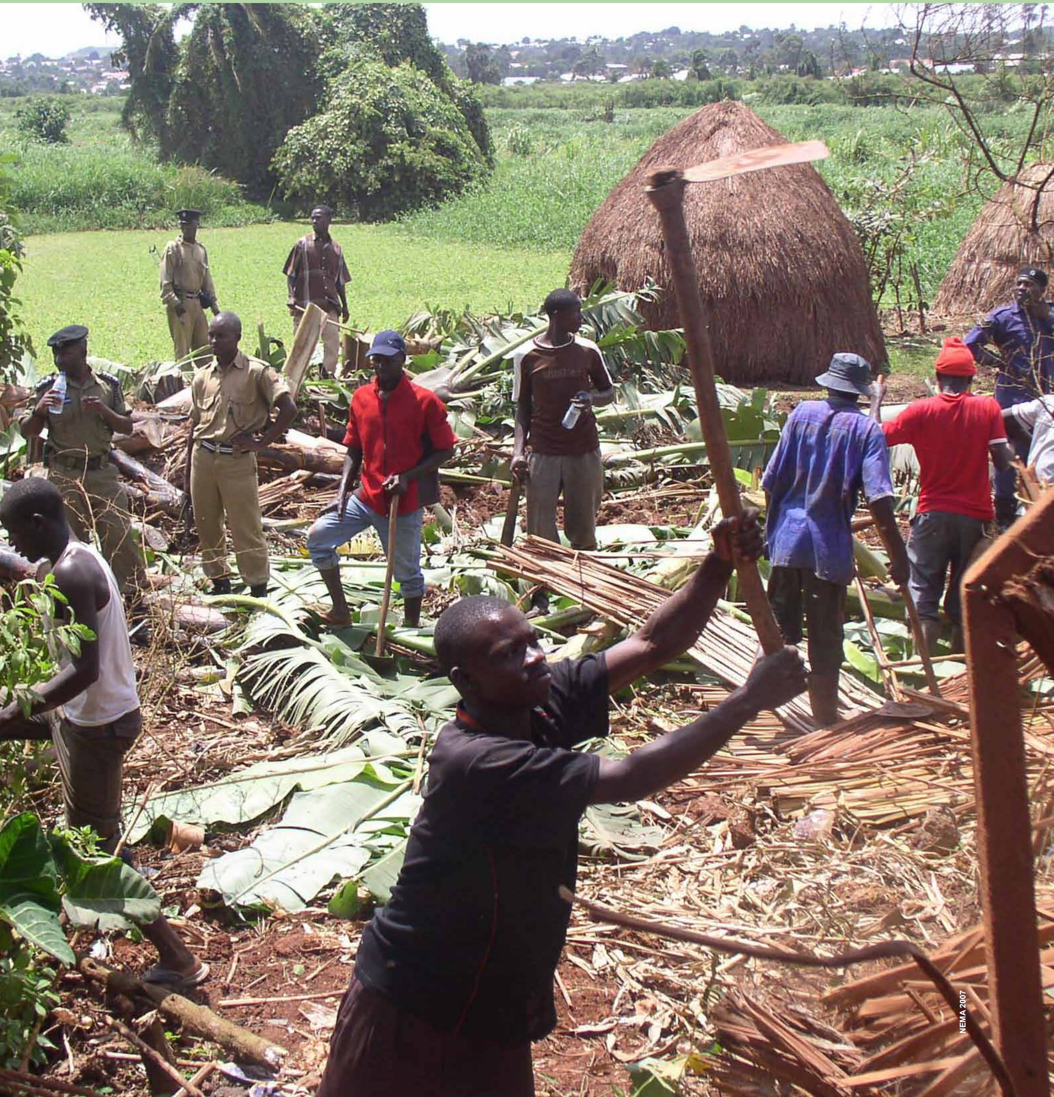
Wetland restoration in progress: Demolition of illegal structures in the Nsooba-Lubigi wetland, a suburb on the outskirts of Kampala City (2009). Enforcement has been intensified in the wake of increased wetland degradation in Kampala and other parts of the country.
