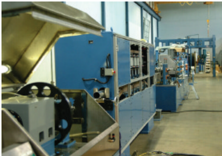
▲ Longitudinal metal tape seam welding and corrugating line
