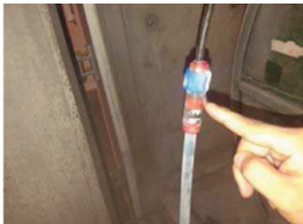
▲ Figure 5: Water frozen around end caps
