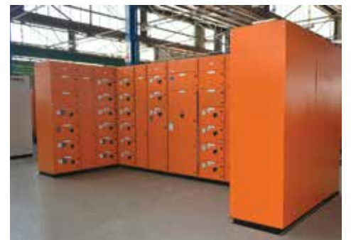
Motor Control Centres
