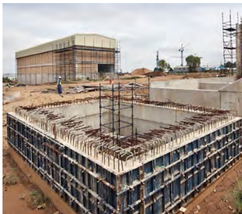
Construction of the new Sebenza substation under way: the three-storey GIS building in the background, in foreground, the oil spill catch pit and to the right, the transformer plinths with fire walls in-between them.
