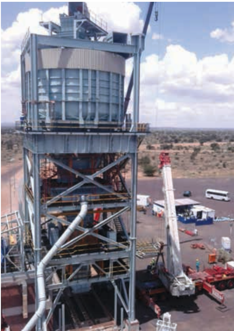
A Rapid Train Loading Station (RTLS) is being provided at Assmang's Black Rock Mining Operations (BRMO).
