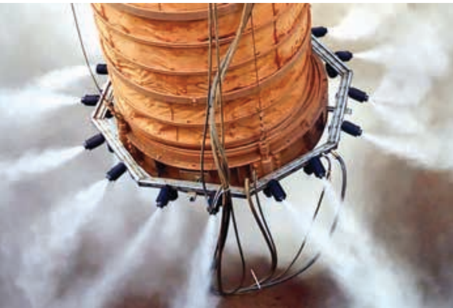
A DSI dry fog system reducing fugitive dust.
