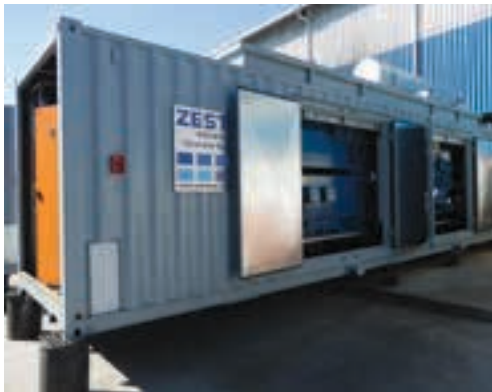
The custom engineered diesel generator set solution for Syrah Resources' Balama graphite project.
