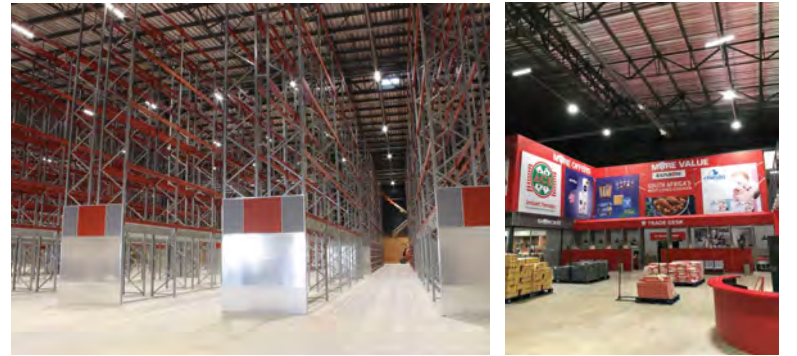
Jumbo Cash & Carry in Crown Mines, JHB features Regent Lighting's Holda 200 W and Thora 200 W suspended from the ceiling between racking to provide the desired light output throughout. Further LED fittings, including the Lugo and Luxon panels, were used throughout the offices and checkout areas while the exterior of the building makes use of the Istria Trunion.
