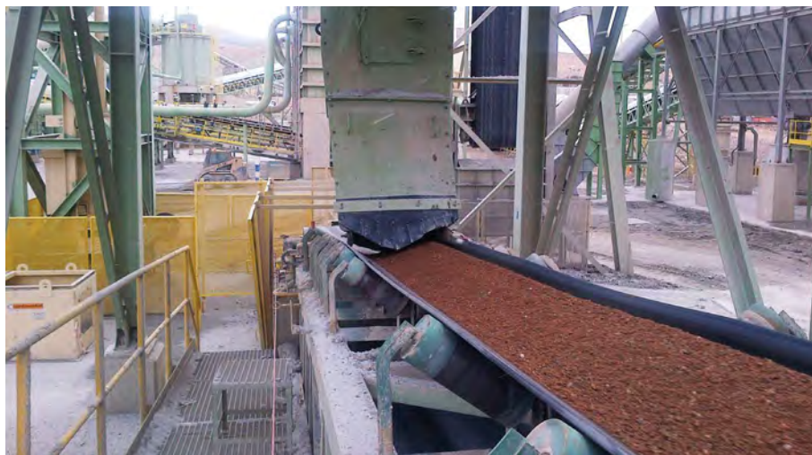
By controlling the fall of material in the transfer point, material degradation can be dramatically decreased by up to 80%, with a resultant decrease in dust and noise emission.
