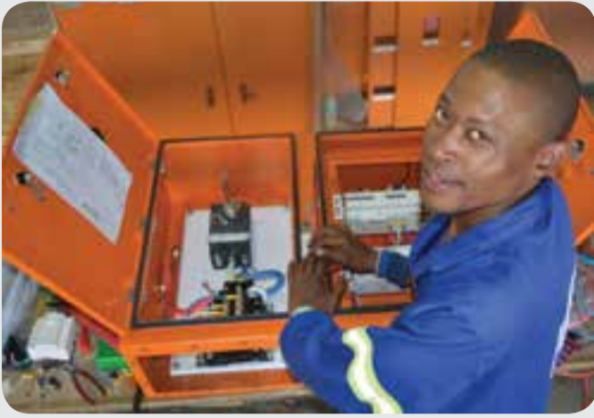
Lebo Ntete in the dedicated electrical workshop for the production of main and sub distribution boards at Shaw Controls.
