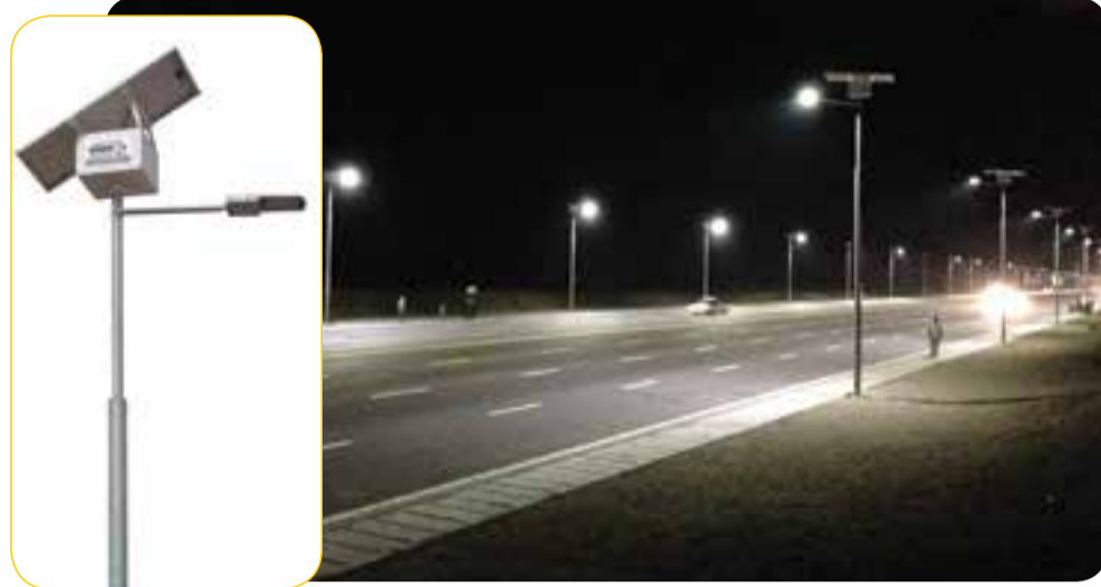
More than 1 000 BEKA Solar units are installed in Kinshasa, lighting up the prestigious main road from the airport to the city.
