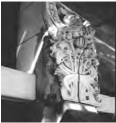
Typical bad repair
