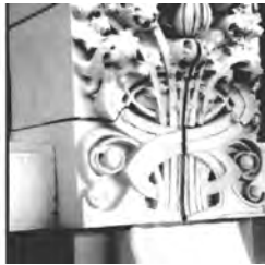
Good blending repair
