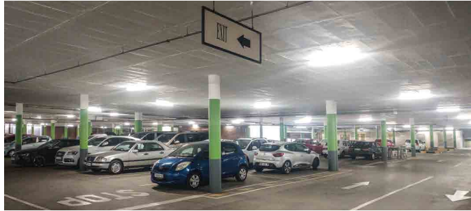
Magnet Energy recently completed the design and installation of a new lighting system at the Centurion Mall's parkade. Advanced lighting technology has significantly improved light levels, enhanced safety and contributed to energy savings.
