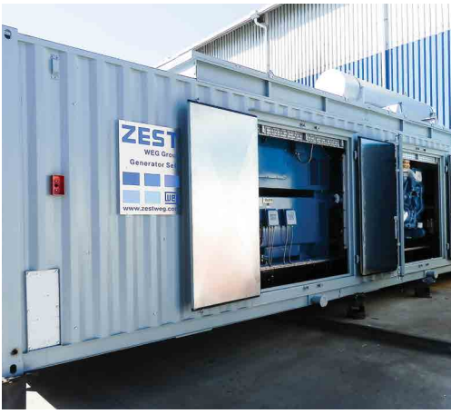
The custom engineered diesel generator set solution for Syrah Resources' Balama graphite project.
