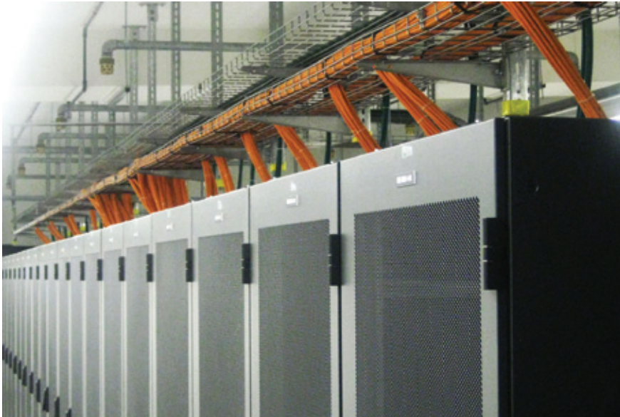
▲ The new data centre from Datwyler
