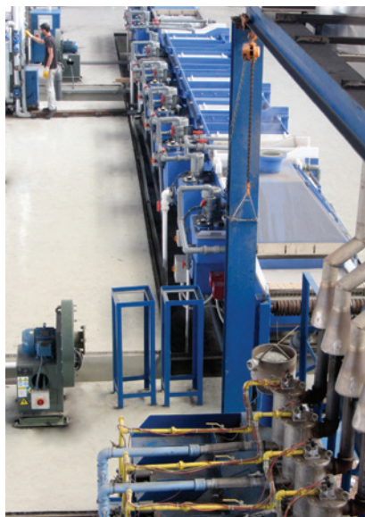
▲ Mark 4 immersion burners on a high carbon line
