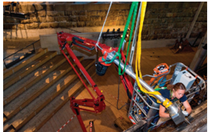
Monika Ash inserts one of the new bolts into an old hole, using a specially built machine
