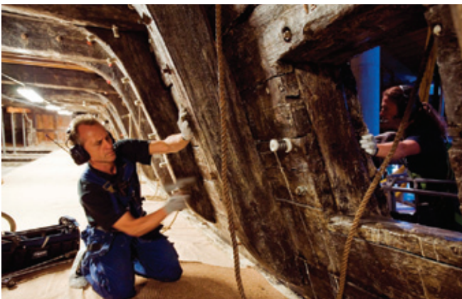
Ove Olsen hammers out one of the old bolts, while communicating with carpenter Monika Ash via radio in the hearing protection headset
