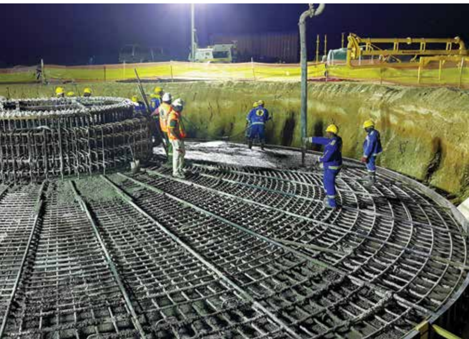
Concor Infrastructure was involved in a number of wind farms including Loeriesfontein and Khobab in the Northern Cape where 122 wind turbine generator foundations were constructed.
