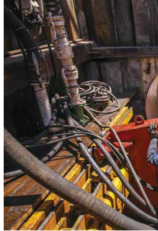
ABOVE: The TBM deployed by CSV Construction was the Herrenknecht AVN 800 XC TBM.
