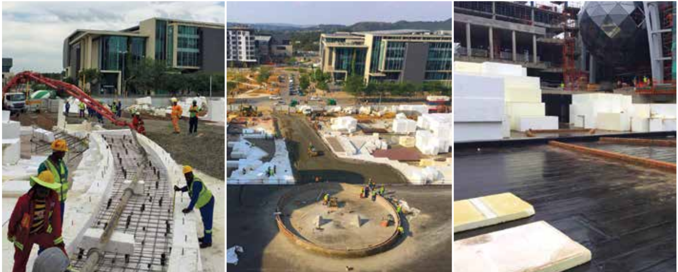
ABOVE: Thusanane Construction Suppliers supplied EPS polystyrene and polyethylene joint formers to the Time Square project in Menlyn.
