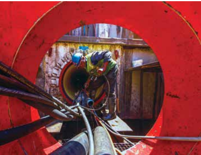
After the TBM has entered the ground from the jacking shaft, special jacking pipes are inserted behind the TBM.
