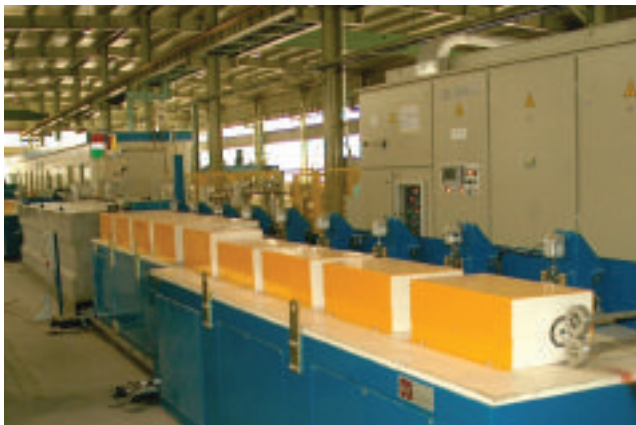
▲ An ATE system installed for Buehler
