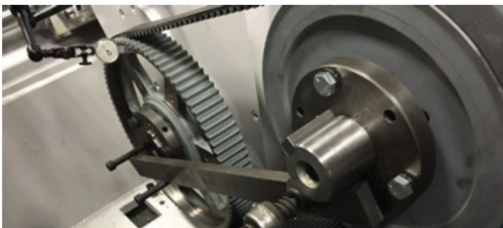
Figure 1: Locked input shaft of the gearbox to prevent rotation
