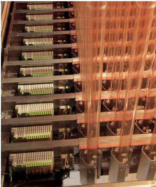
The compact electronics that control the 529 Plexiglas tubes are installed at both ends of the support structure. The controls consist of an EK1100 EtherCAT Coupler, digital input terminals, servo terminals, and buffer capacitor terminals.
