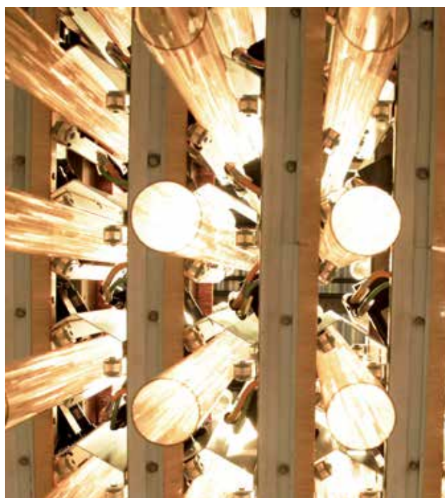
A total of 529 AM8121 servomotors and 529 EL7201 servo terminals were installed in order to move all the Plexiglas tubes.
