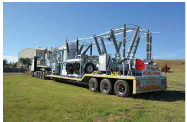
132 kV/88 kV//33 kV/22 kV, 40 MVA multi-ratio mobile substation set up for transport mode and ready for deployment to the operational site.
