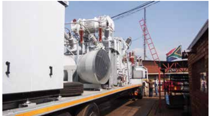
An ODAF (Oil Directed Air Forced) cooling system is utilised to minimise the physical size and overall weight of the transformer.
