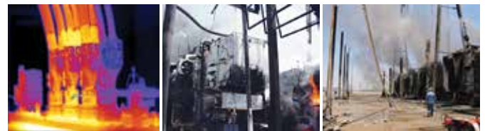
Figure 2: Degradation of assets occurs in the form of heating of cables, insulation degradation, cooling fan problems, tripping of VSDs during unbalance conditions which ultimately result in damage to equipment and reduction of asset lifecycle.
