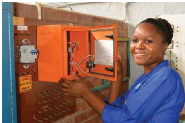
Veronica Ramashala, Level 3 electrical infrastructure learner at Tshwane North TVET College during a practical lecture demonstrating the WG MDWH miniature circuit breaker.
