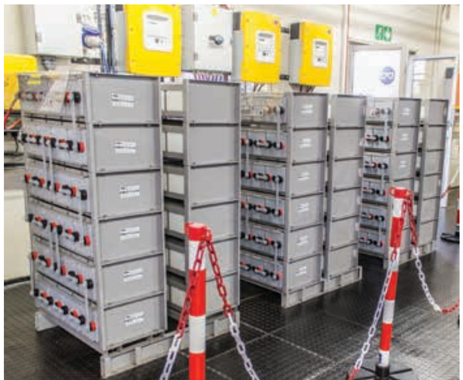
Battery storage capacity of 120 kWh is used to store PV-generated power for use by the electrolysers and hydrogen pumps, while SMA inverters make ac power available to the centre.
