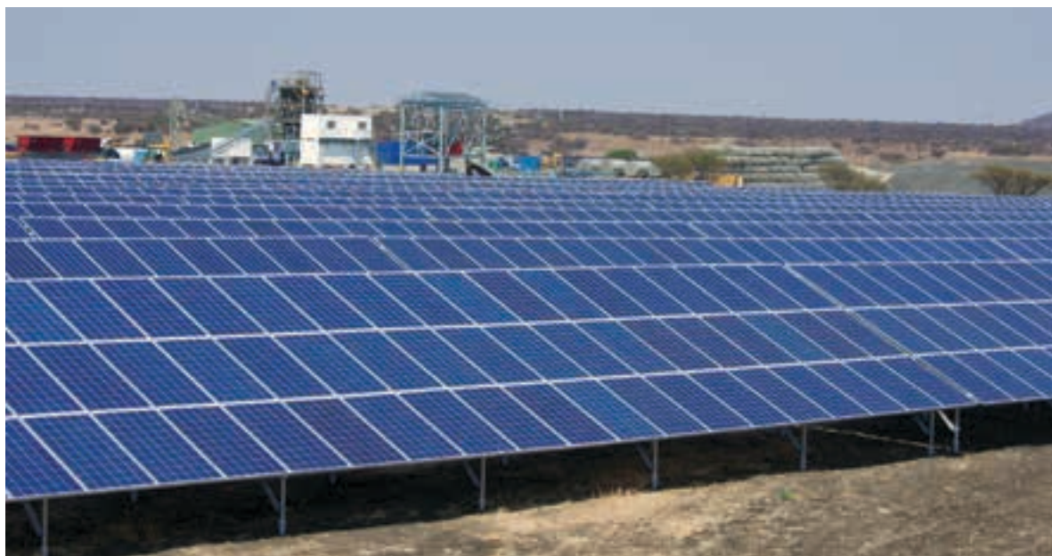
A recent study, 'Low-load Gensets for Solar-diesel Hybrid Plants in the Mining Industry' shows that low-load gensets almost double the solar penetration rate in solar-diesel hybrid systems and that low-load diesel gensets are more efficient in hybrid plants.
