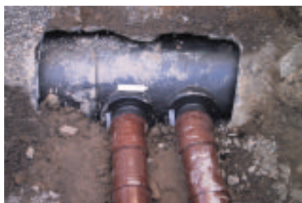
▲ The connection of PE 80 external saddles for service pipe connection to the main sewer and a PVC-KG pipe
