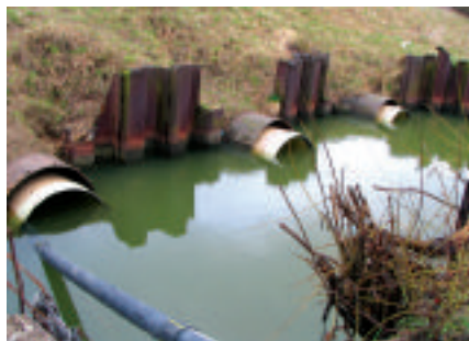
▲ HOBAS DN 1200 pipes were used to rehabilitate three parallel culverts into which the sewer main divided to fit under a railway
