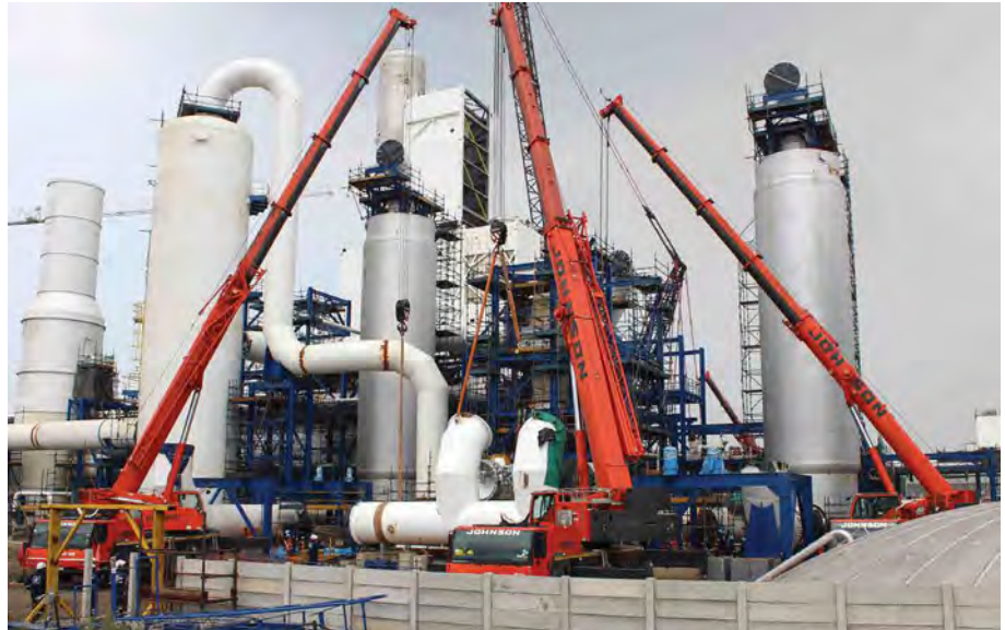
Close attention to planning and safety procedures were key to the smooth implementation of the lifting project.
