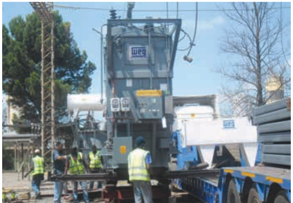
An important value-added service offering from WTA is its suite of structured transformer maintenance programmes that allow customers to protect these assets from degradation.
