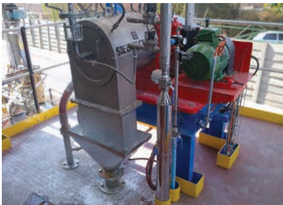
A Conturbex centrifuge dewatering glauber salt product in a ZLD plant.
