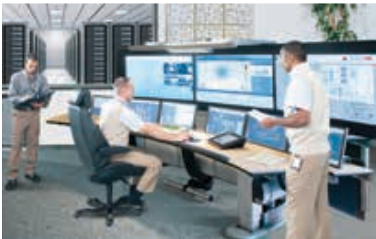
Located on centennial campus of North Carolina State University, this state-of-the-art Smart Grid Centre of Excellence (COE) has functional systems where information technologies (IT) and operational technologies (OT) converge to close the loop of automation, control, data acquisition and asset management.
