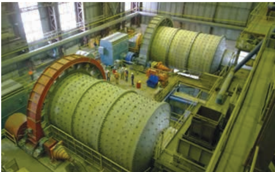
The FLSmidth ball mills at Zangezur Copper Molybdenum Combine (ZCMC) in Armenia. The second mill was recently installed using the company's recently introduced Super Supervision service.
