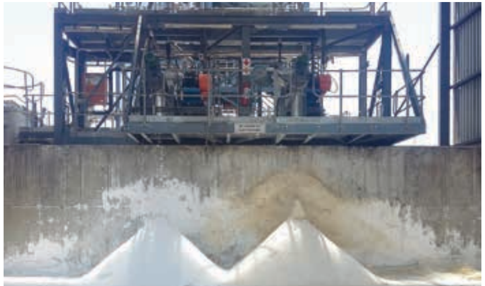
Two Conturbex centrifuge installations dewatering glaubersalt and mixed salts produced using a ZLD process.
