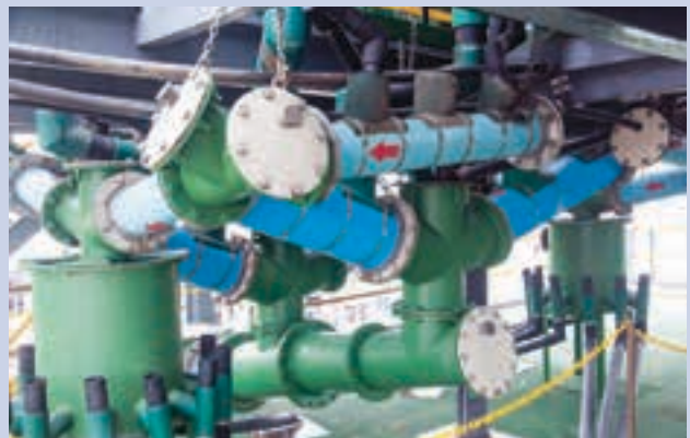
The cleaner concentrate, rougher concentrate and tail pipe launder arrangement, together with Multotec distributors.
