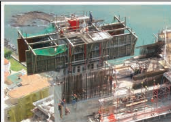
Climbing, shuttering and safety systems with independent controls of 200 ton platforms. Trump Towers, Panama City.
