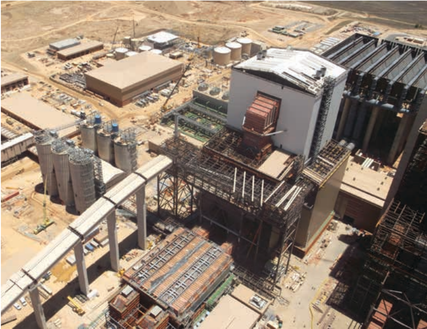
A view of the nearly completed Unit 1 boiler at Kusile, the site of ABB's flagship control and instrumentation (C&I) project.
