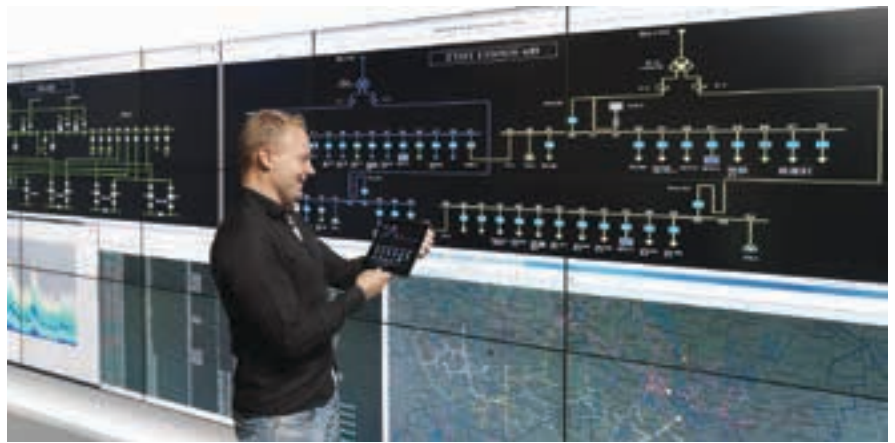
"Internationally, ABB is Number 1 in C&I, says Viljoen. "We are unique in this field in that we don't manufacture the mechanical equipment such as boilers and turbines, so we have the ability and experience to customise control solutions that are robust and flexible, regardless of which OEM's equipment it involved."
