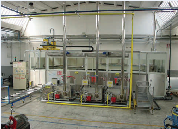
Figure 15: Automatic equipment (outer and inner) for ultrasonic cleaning, rinsing, passivation and drying of carbon steel tubes for air conditioning and heating plants
