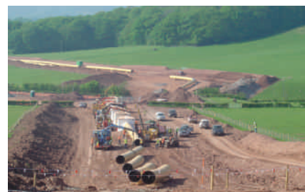
The early stages of another X80 project in the UK: the start of 48" X80 mainline welding for Murphy in South Wales
