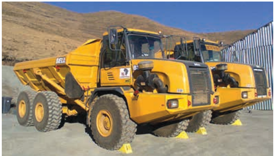
Bell ADTs from Turnkey Civils Lesotho (TCL), shortly after arriving on site. TCL is the contractor for the Residue Storage Facility (RSF) and moved on to site in June last year.
