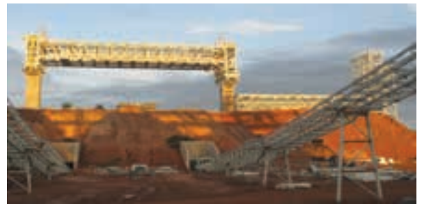
The first 1 200-tonne prefabricated conveyor truss in position at First Quantum Mineral's Sentinel copper mine near Mwinilunga in north-west Zambia.
