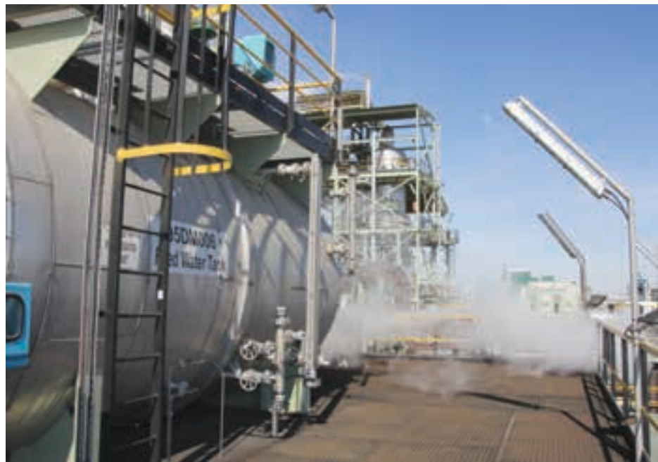
A section of Omnia's new nitric acid plant with the ammonium nitrate plant in the background. Hay views the plant as a strategic asset that will give Omnia and BME a competitive edge for years.
