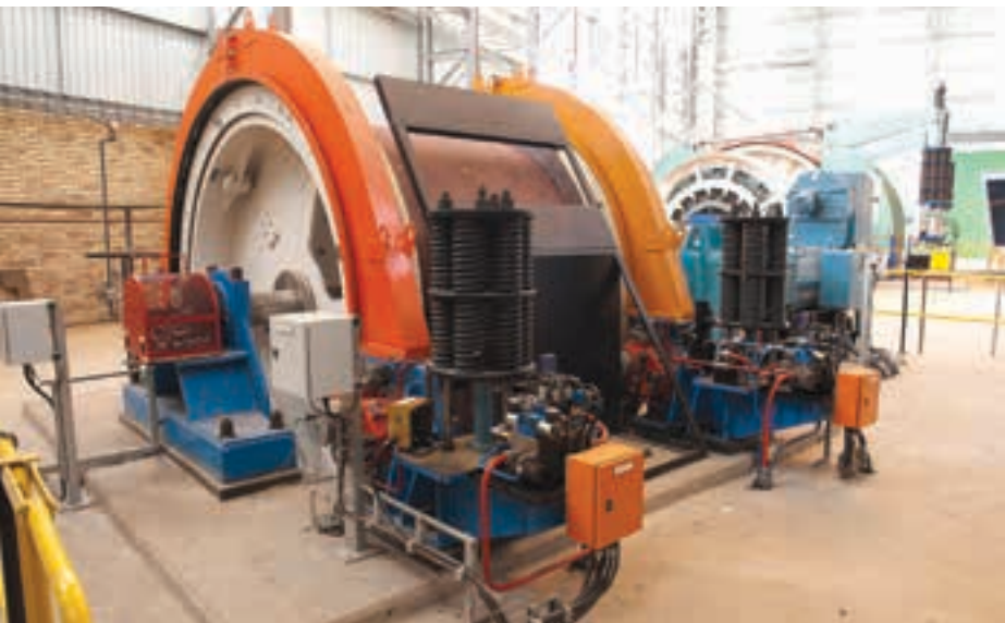
Inside the main shaft winder house. Bakubung's total hoisting capacity is 265 000 tonnes/month.
