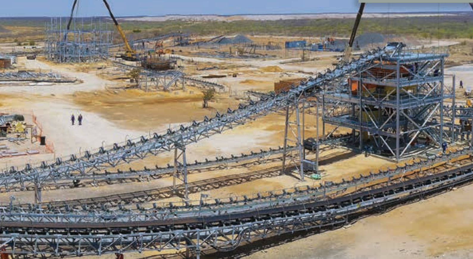
The Karowe site (in September 2014) showing new conveyors in the foreground, the final recovery building in the distance and (to the right) the XRT plant under construction (photo: Arthur Tassell).
