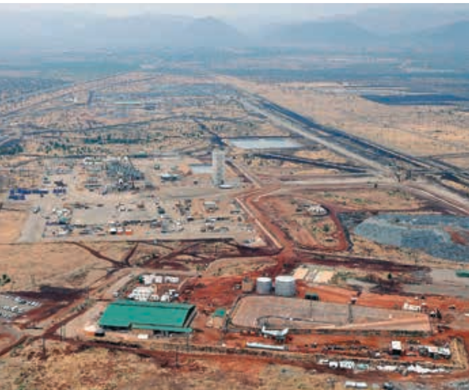
Above: Aerial view of the Project 1 site. As at the end of November, the project had reached 70 % completion.
