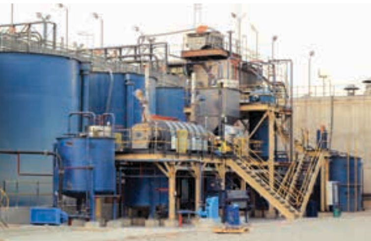
An ADR plant supplied by FLSmidth for Shanta's New Luika Gold Mine in Tanzania is exceeding the design performance target.
