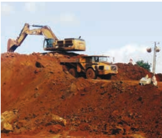
The Tokadeh iron ore mine near Yekepa in Nimba County in Liberia, where the Zest WEG Group's Enl Electrical is responsible for all overhead line infrastructure.
