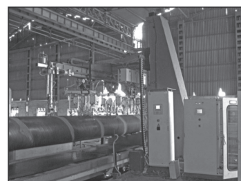
Spiral Pipe Testing System
