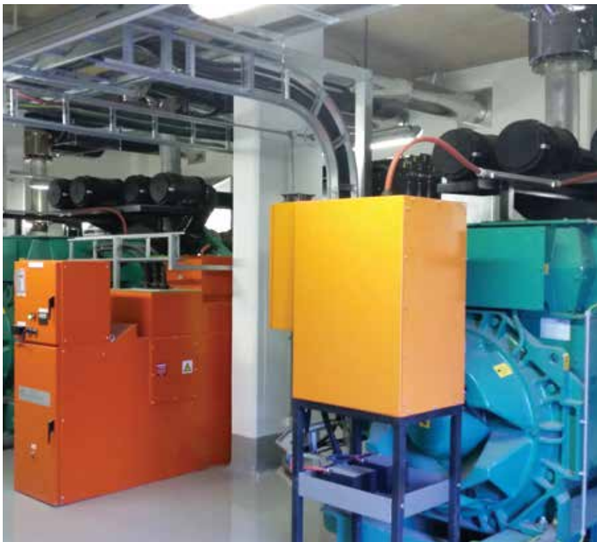
Cummins supplied SABMiller Alrode Brewery with four C2500 D5A diesel generator sets for emergency standby power. The 6,6 kV generators boast a prime rating of 1 800 kVA, and are powered by a Cummins QSK60G8 engines.
