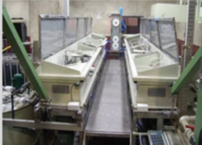
Electrolytic tinning plant (waste water free)
