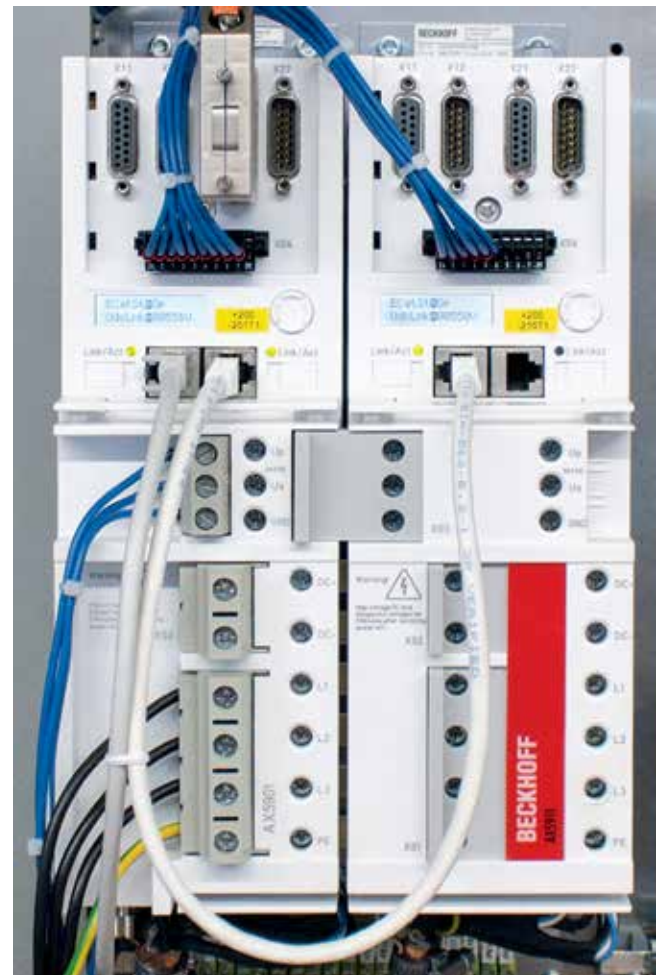
Two AX5206 Servo Drives with AX5805 TwinSAFE option cards control the AM8000 OCT servomotors. Copyright: Bauer Steuerungstechnik, Germany
