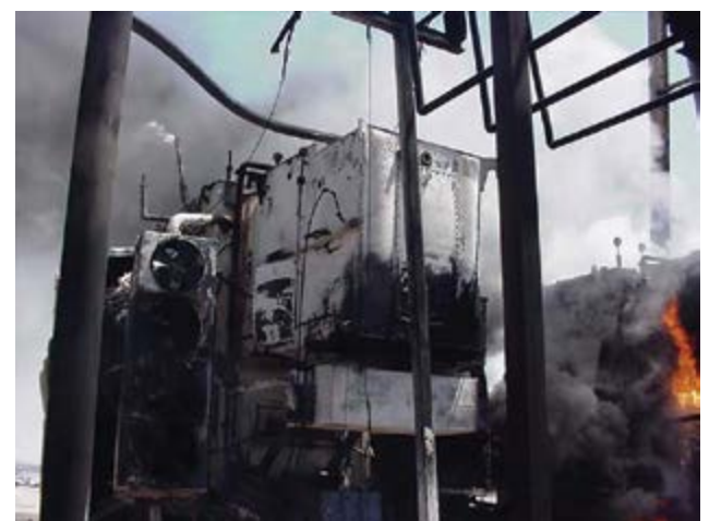
Catastrophic transformer failures are possible.
