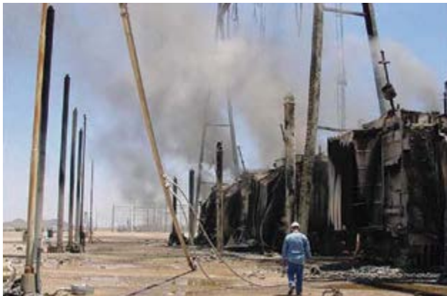
Transformer failure – costly clean-ups and recovery.
