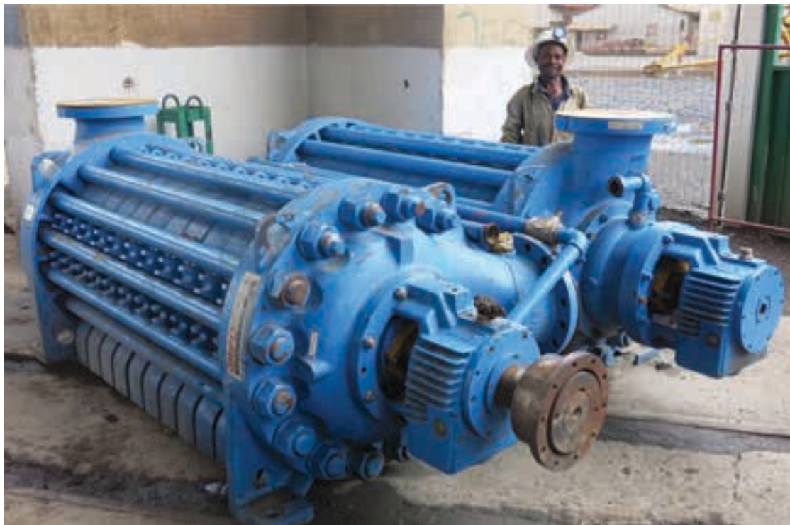
Two of three new high-volume Grifo pumps to be installed at the main pumping station 1 210 m below surface (photo: Ivanhoe).
