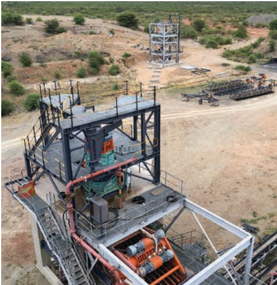
The new Kawasaki secondary cone crusher (foreground) with the relocated surge bin and conveyor plinths in the background (photo: Kimberley Diamonds).
