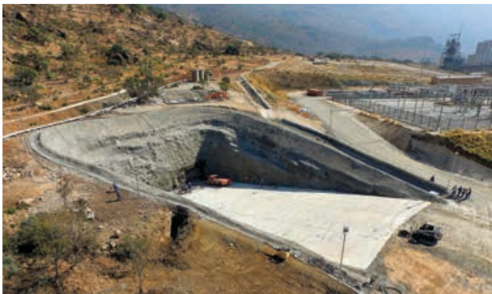
The Merensky boxcut during construction. Note the proximity of the Eskom substation.
