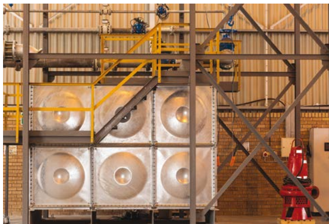
A front view of Integrated Pump Technology's new 90 kW test tank facility, commissioned at its Johannesburg premises.
