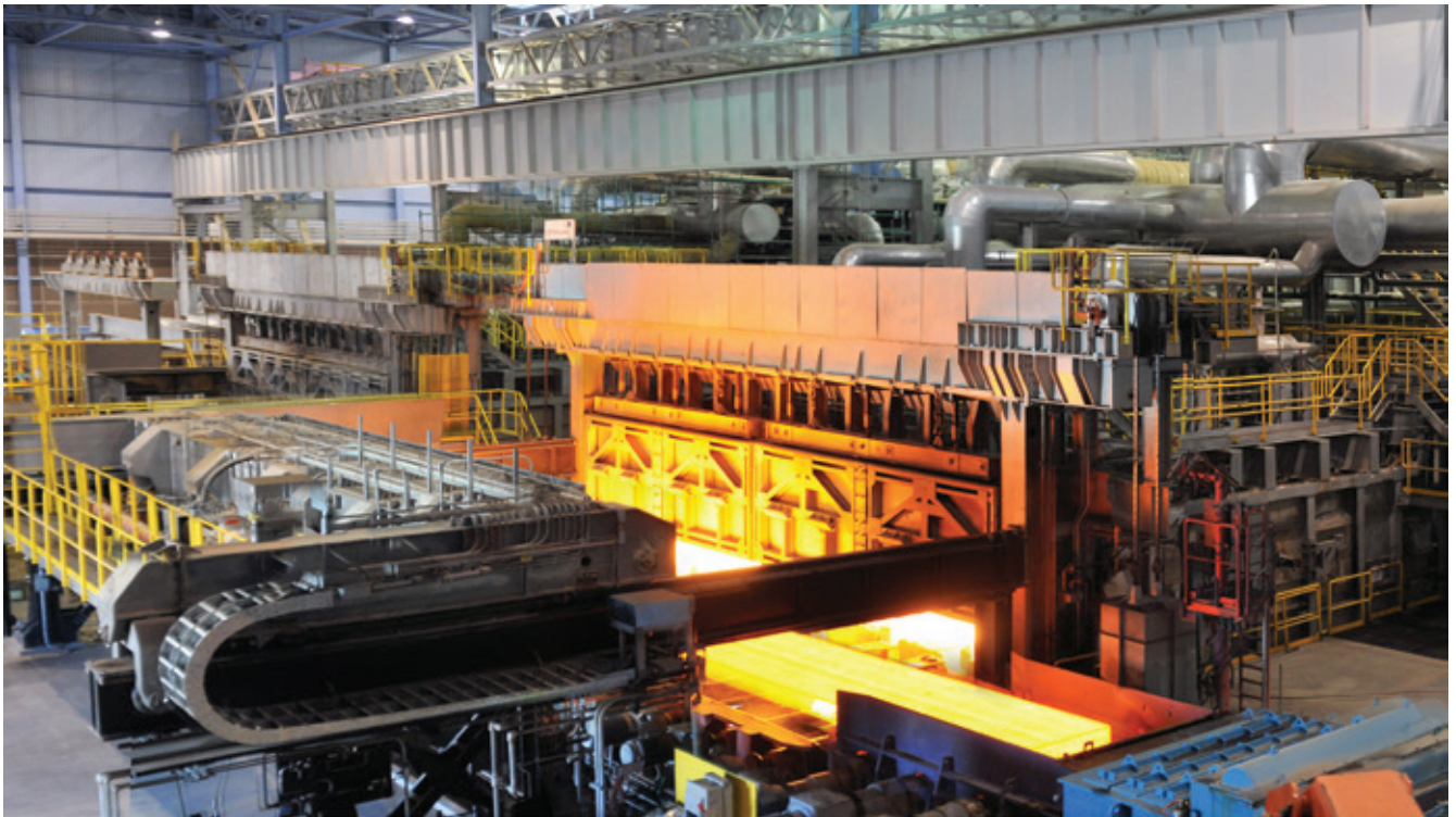
○ A walking beam furnace from Tenova
