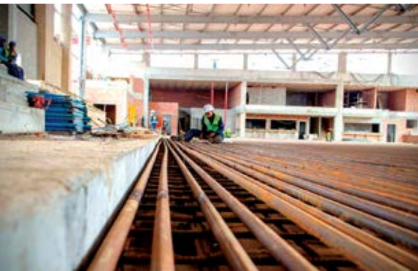
Workers carefully lay the piping which forms the foundation of the 2 300 m 2 Baywest ice rink in the mall’s R100-million Fun Factory wing. The mall will open this April, upon which time development around the centre to the value of R500-million will commence.
