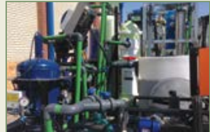
Mobile filtration system.
