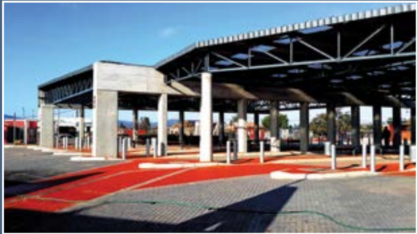
Lafarge Agilia™ concrete was used to construct South Africa's first green taxi rank in Cape Town.
