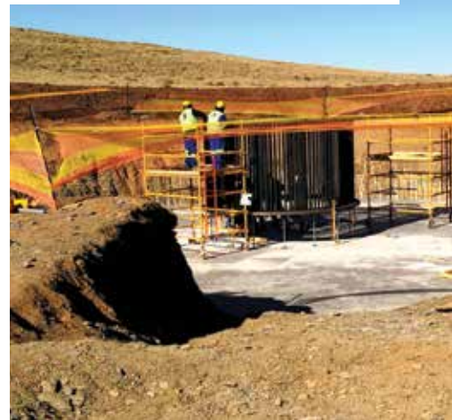
Bolt pack erection after pouring blinding on one of the wind turbine bases at Noupoort Wind Farm.
