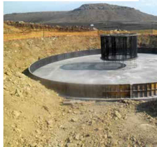
Erection of the bolt pack after blinding has been poured at Platform 24 at Noupoort Wind Farm.
