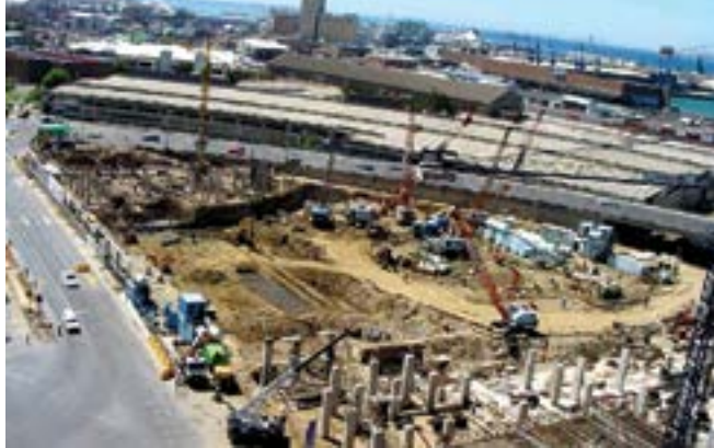
Franki Africa has been contracted to implement a range of geotechnical work on the Cape Town International Conference Centre (CTICC) East Expansion project.
