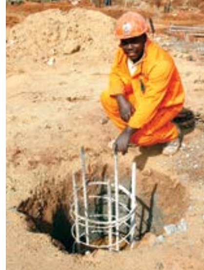
Gauteng Piling site foreman, Tshifhiwa Ndwambi, pictured at one of the 91 piles the company provided for a new Sasani Studios building at Highlands North.
