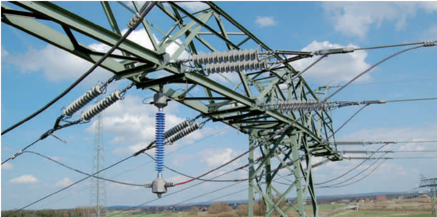
▲ Figure 11: Completely assembled temperature and strain monitoring system
