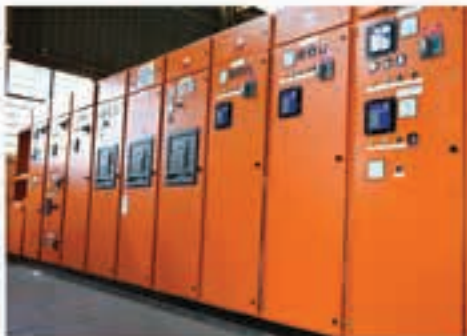
SC100 Motor Control Centre
