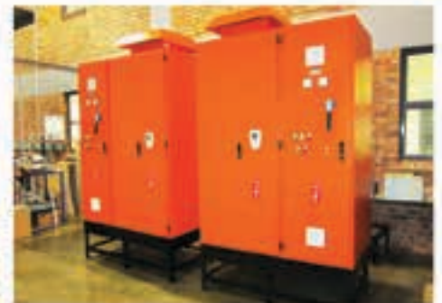
CFW Family Variable Speed Drive
