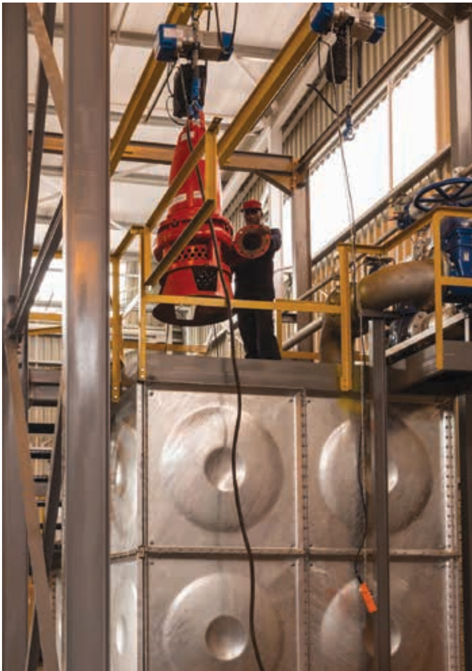
The 18 000 litre test tank measures 3.6 m by 2.4 m and is fully automated, with different programs for specific Grindex pumps, which are tested according to the OEM's pump curve.
