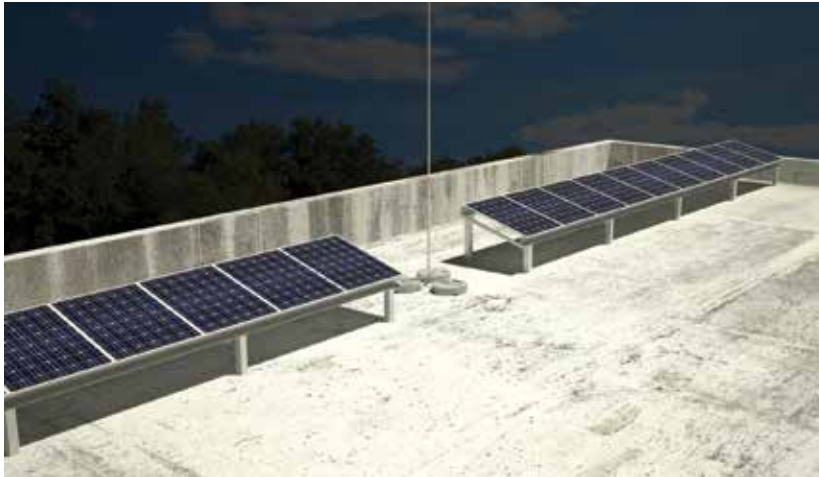
Self supporting air-termination rod.
