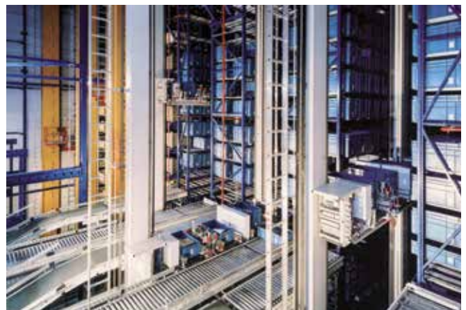
The use of safety laser scanners from Leuze ensures protection of workers in automated plants.
