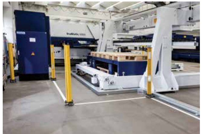
The Leuze MLD safety devices have six different muting operating modes.
