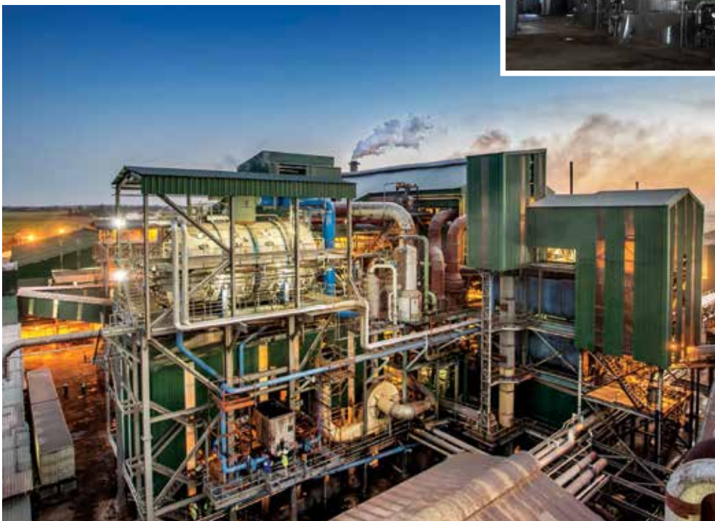
The Nakambala Product Alignment and Refinery (PAAR) project at Nakambala Sugar Mill in Mazabuka, Zambia, is one of the largest projects Bosch Projects has undertaken to date.
