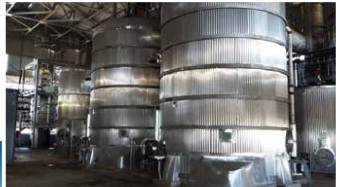
Completed refinery with a view of the conditioning silo supplied by Bosch Projects.
