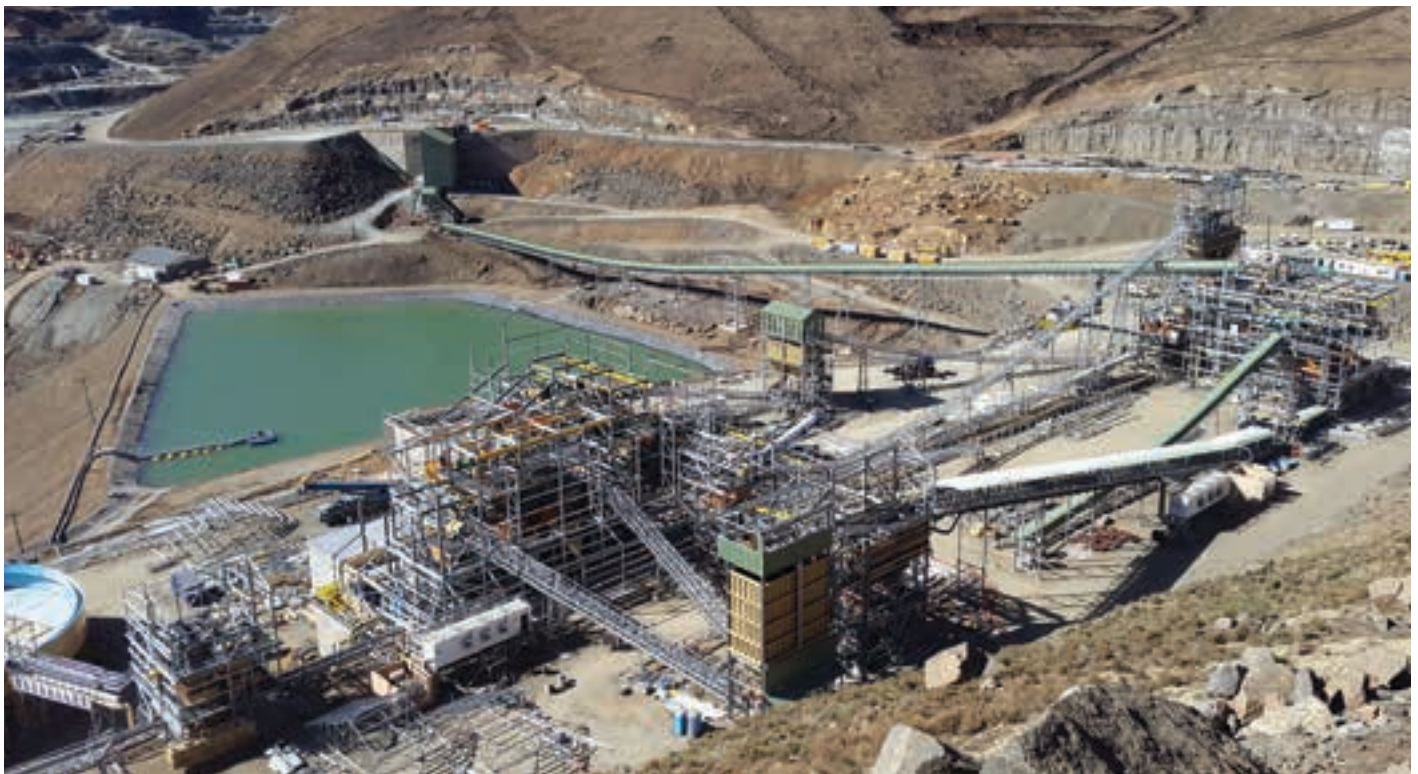
Construction work on the main plant terrace at Lihobong (photo: Firestone Diamonds).
