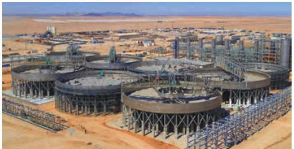
FLSmidth 40 m diameter CCD thickeners installed for Swakop Uranium.
