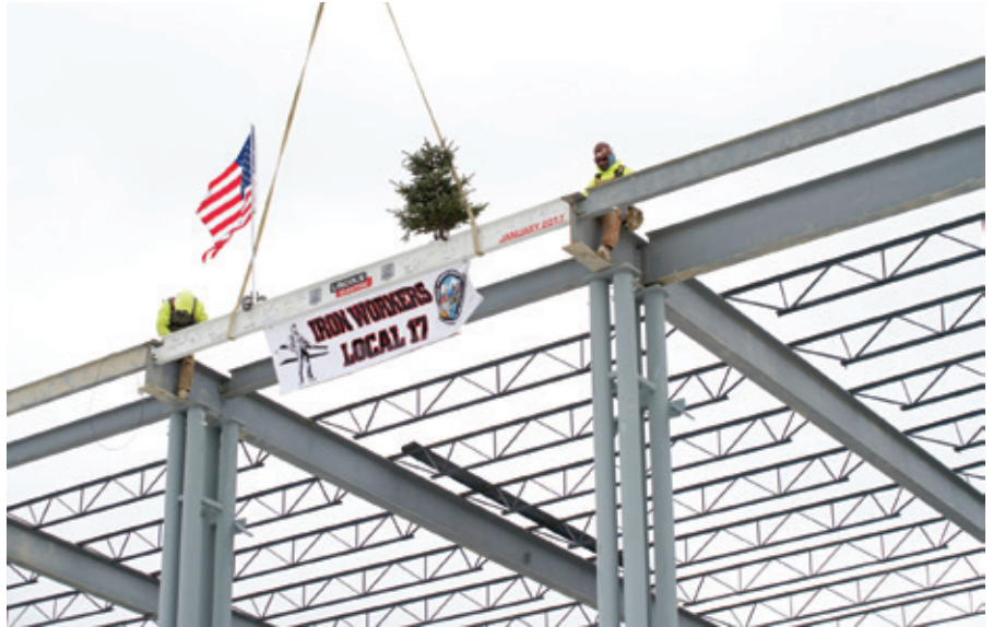
Crews placed the final beam of Lincoln Electric's new Welding Technology Center
